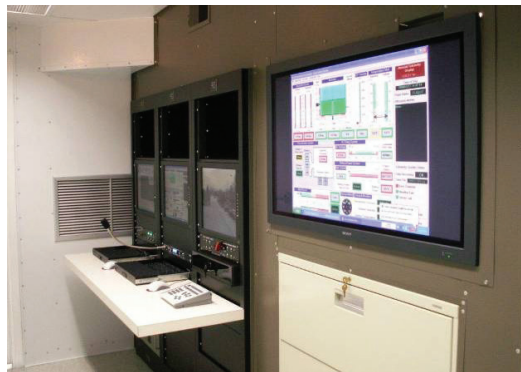
Gambar 6. Ground Control Shelter (LEN, 2016)
